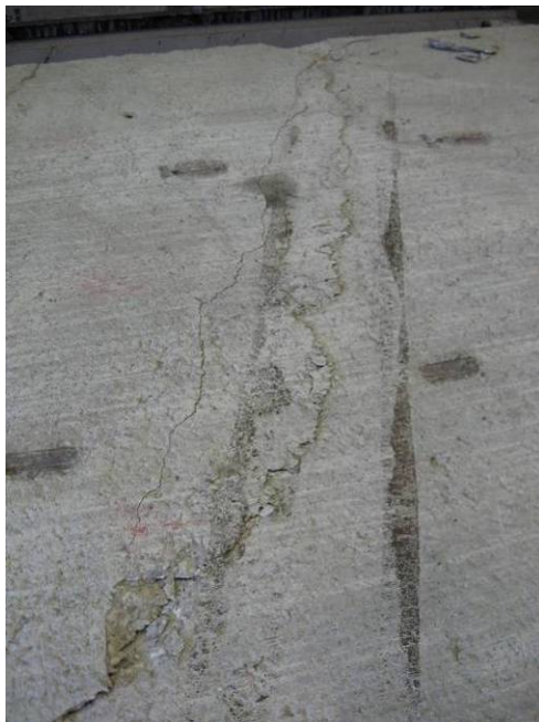
Figure 3.30. Flexural cracking in deck panel due to applied line load.
